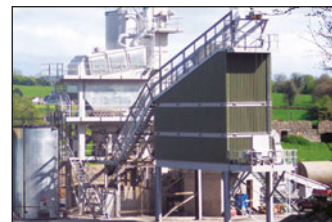
210 tonne mixed material storage - Ireland
