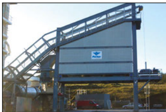
210 tonne hot mix storage capacity, 3 x silos - Northern Ireland
