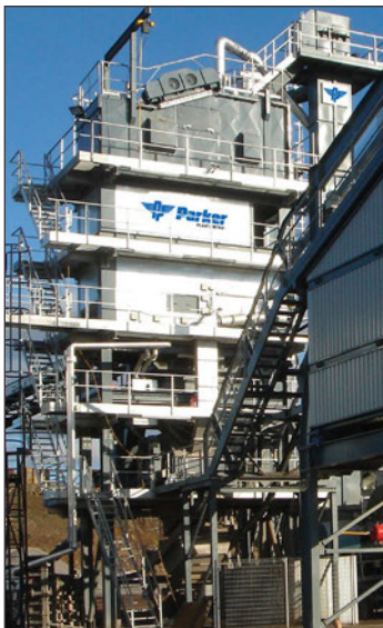
Note: Bag Filter Specification listed separated
